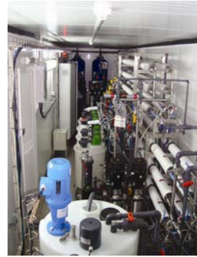
NEEMEA Water treatment for a Power Plant in Kenya
