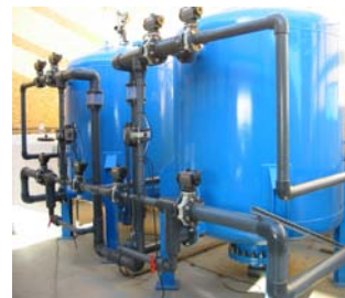
NEEMEA – Water treatment for an ecological camping site (Portugal)
